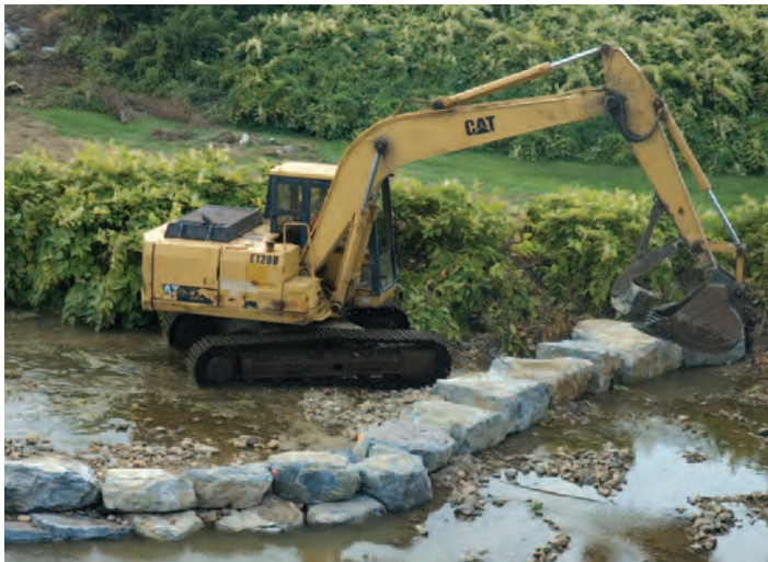
Conservation grants from the Virginia Fly Fishing Festival Foundation helped pay for these stones, which are excellent structure for the local trout. Photo by Beau Beasley.
